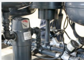
Air Filter - Pic. 5
