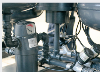
Air Filter - Pic. 5
