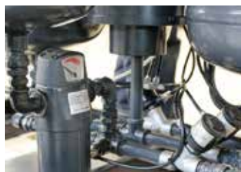
Air Filter - Pic. 5
